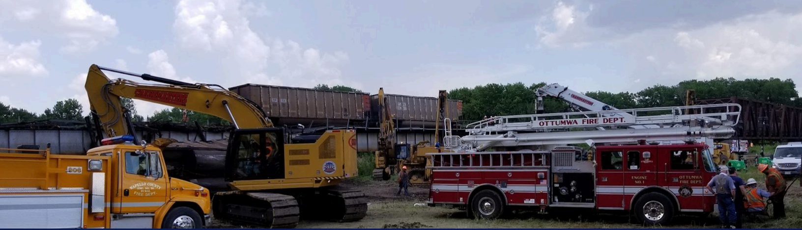
County crews, Ottumwa Fire, and contractors working a rail incident together.
